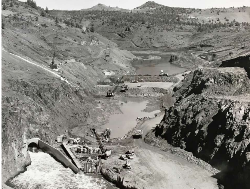
Figure D-10. View Looking Upstream at Site of Iron Gate Dam during Construction and Showing Reservoir Area
